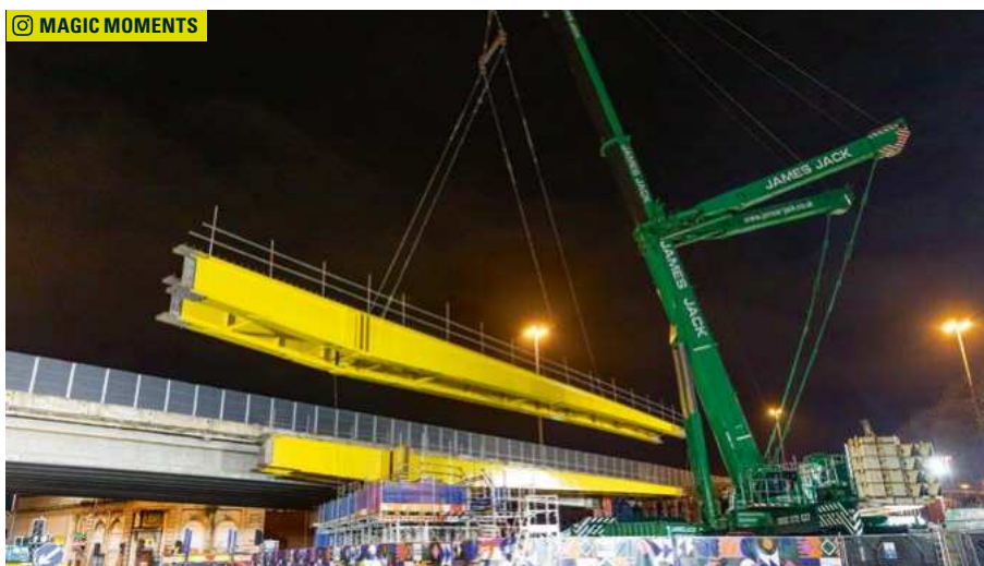
UK: Regent Street bridge lift, Leeds City Council. Photo credit: Catherine Morgan
