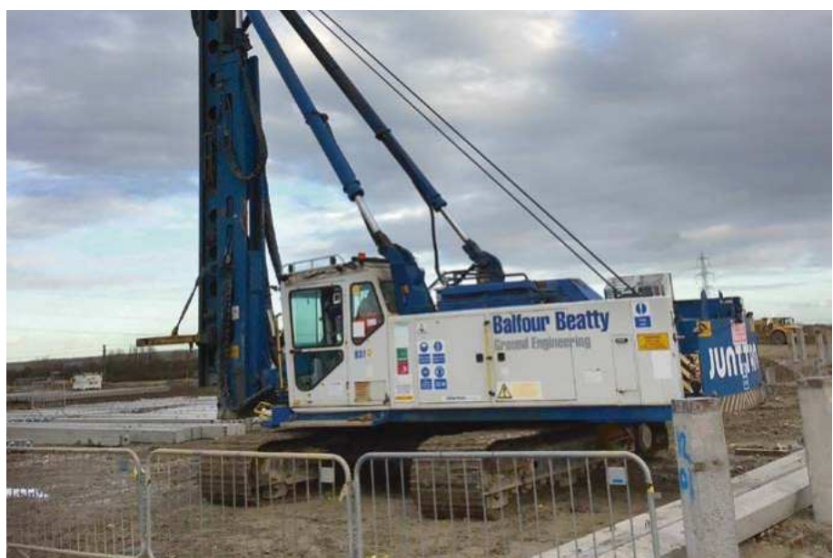
ABOVE First EU Stage V equivalent retrofit project on a Junttan piling rig
