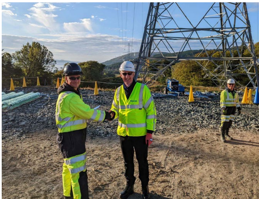
ABOVE: Leo's site visit to SSEN Transmission's Port Ann to Crossaig overhead line project in Scotland.
