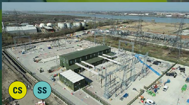
Littlebrook substation, Kent, UK
