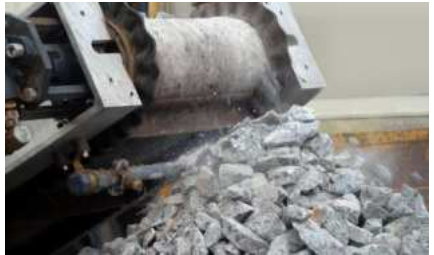
Recycled or re-used 90% of waste materials reconstructing footways using circular economy principles in Lincolnshire
