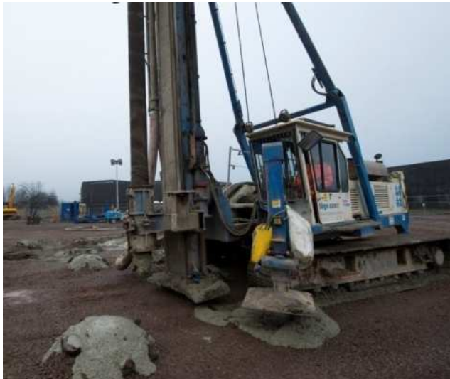
SOME HEAVE DURING INSTALLATION PROCESS
