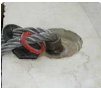
Wire slings bent over!
