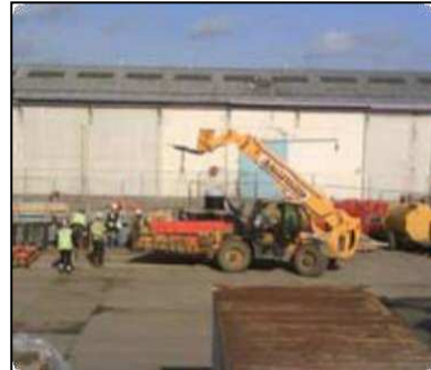
Attachment and load incorrectly positioned
