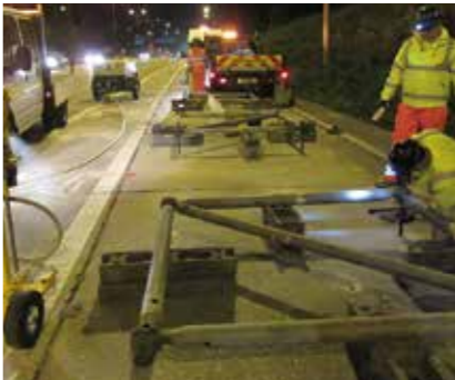
Stage 2 - Resin anchored sockets are installed and holes are drilled for grouting
